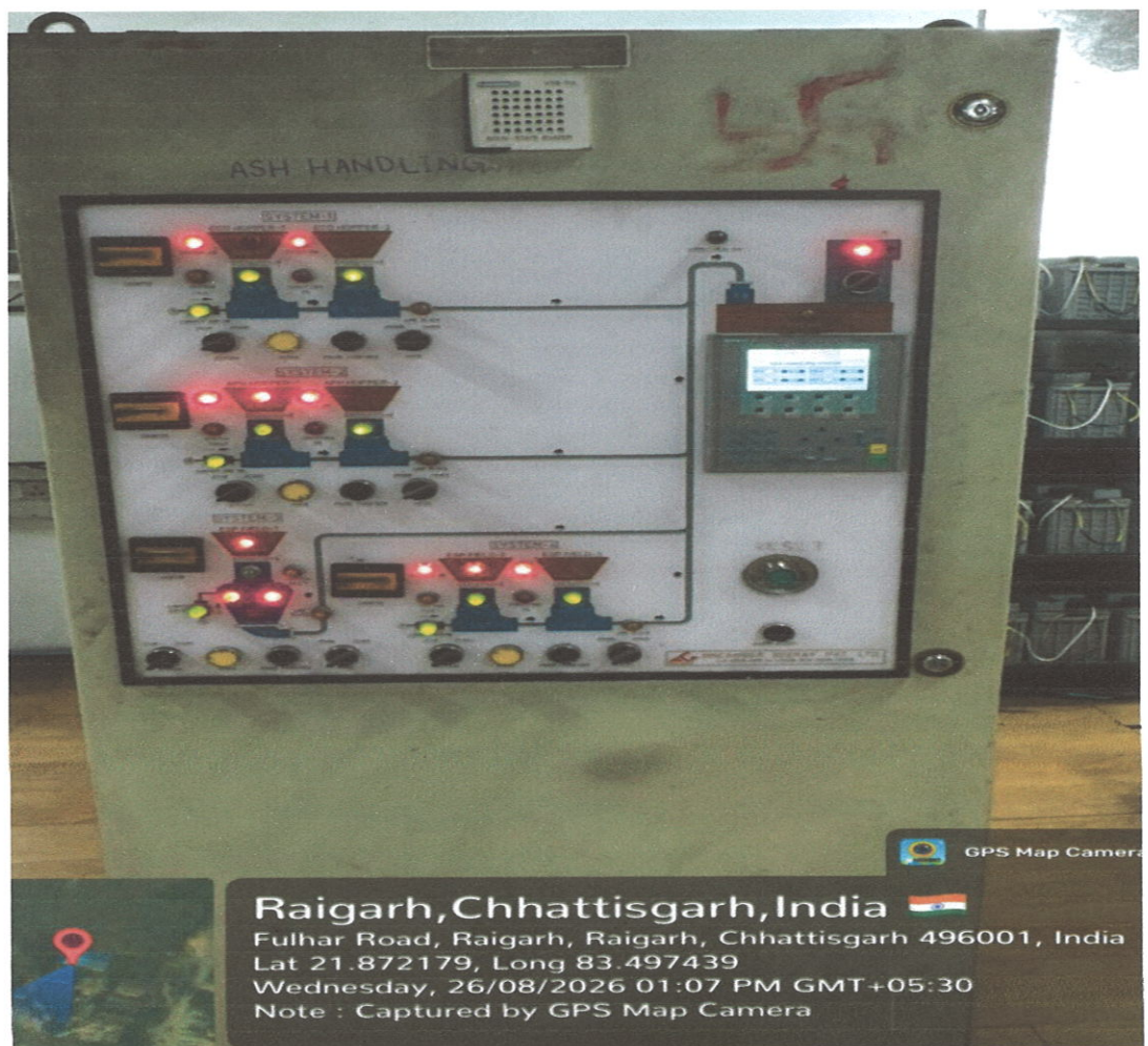
Figure – 10, Ash Handling panel
